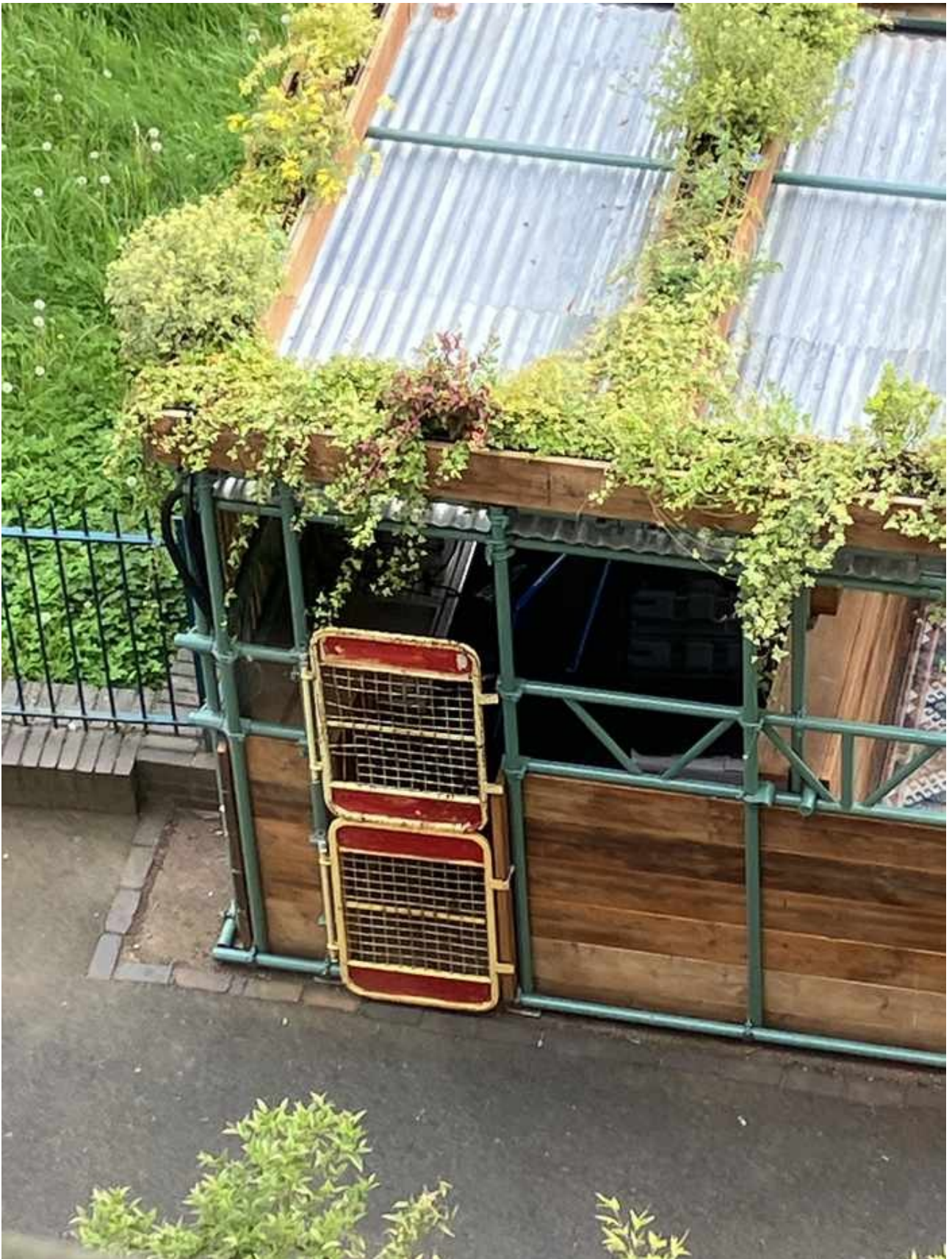
Photograph 2: Close-up structural detail showing the corrugated metal roof section, solid timber planking, and green metal scaffolding poles — all acoustically reflective materials.
